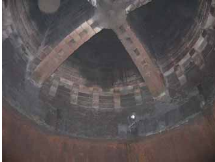
Figure 3 – EPIC Gasifier Internal Refractory 2
