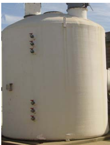
Figure 11. Mercury Adsorption Bed (Courtesy of US Filter)
